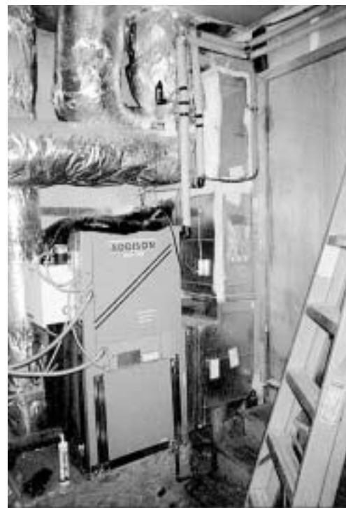
(below) Mastic sealing on central air distribution plenum next to GSHP
