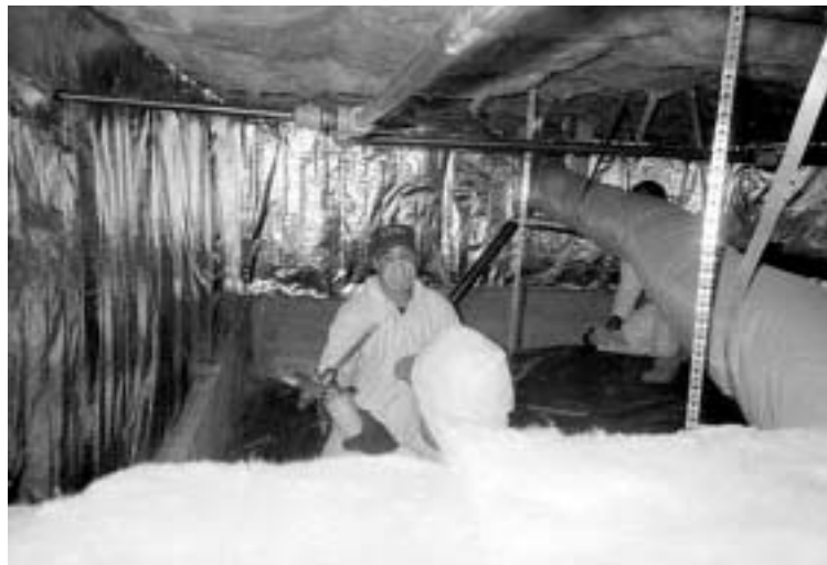
(above) Foam insulation in a crawlspace about to be applied between foundation wall and knee wall
