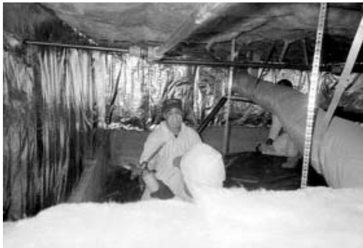
(above) Foam insulation in a can about to be applied between foundation wall and knee wall
